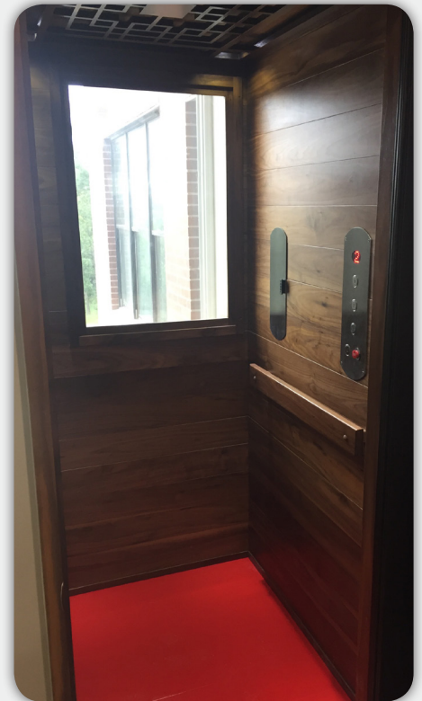
Residential elevator with custom faux shiplap panels and an upper window
